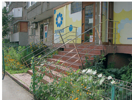
9, From grey to colorful; from cold to warm. A ‘communist’ block of flats undergoing refurbishment and thermal insulation.
